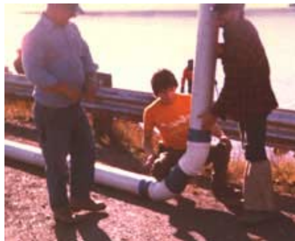
Photo 2: Gluing riser section on the assembled horizontal run section. Note the wide sweep elbow.
