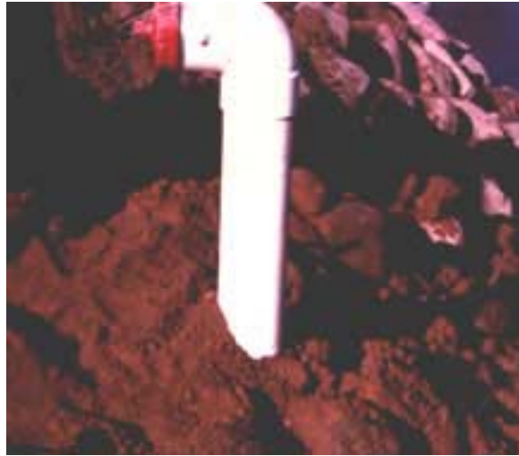
Photo 6: Top of riser pipe temporarily covered with hydrant connection to prevent fill material from entering pipe.
