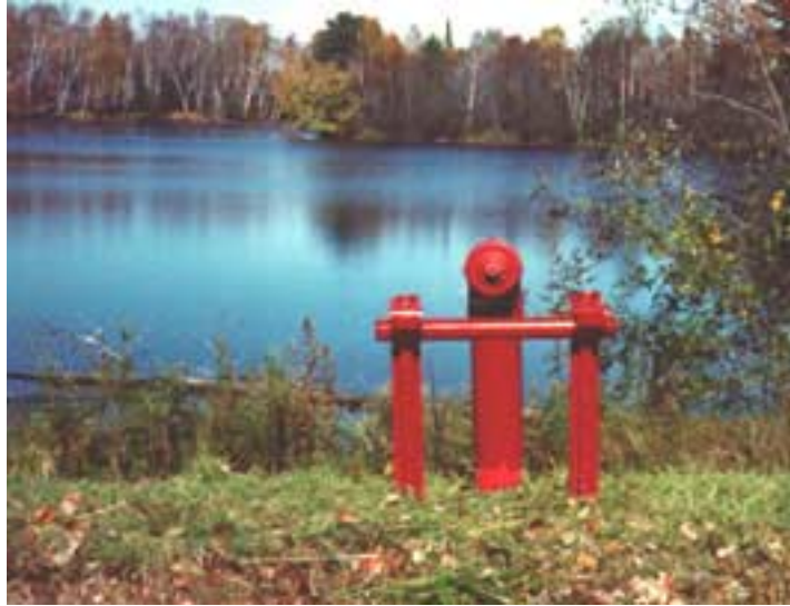
Photo 9: Completed hydrant installation with guards and suction hose support installed. Area has been seeded and mulched to prevent erosion.
